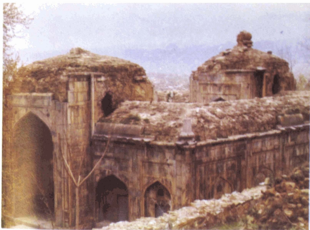
12. The Akhund Mullah Shah mosque, built by Dara Shikoh. Once faced in grey limestone, this exquisite building is rapidly falling into ruin.
